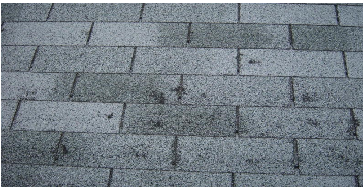
Hail damage caused by severe storms in eastern Nebraska
