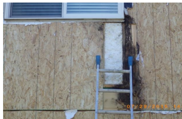
Water Infiltration at Window
