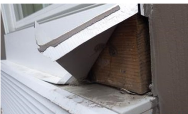
Missing Flashing at HVAC Unit
