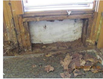
Rotting Due to Water Intrusion
