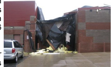
Wind Damage to Roof from Improper Membrane Termination
