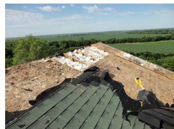
Roof Damage caused by Improper Attic Ventilation
